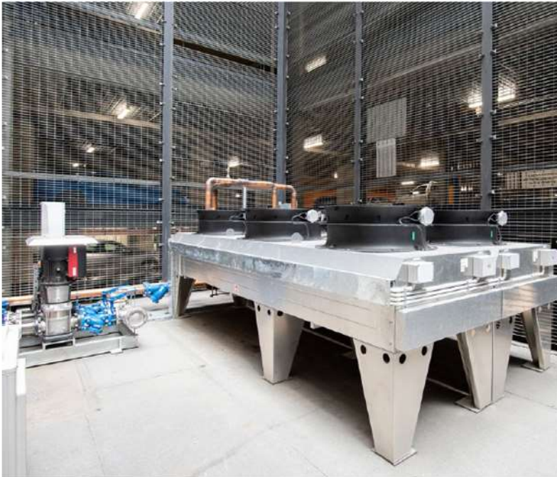
LEFT Machine room, Melbourne store.
